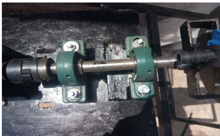
Fig.5. Shaft Arrangement between the motor and PVC pipe
